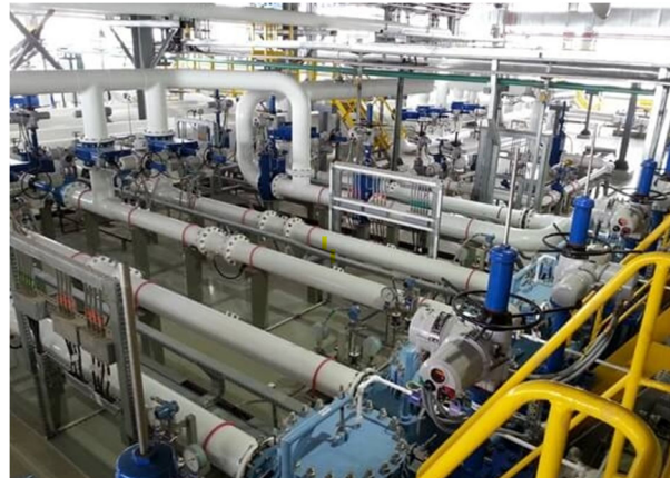
A petroleum liquid processing facility
